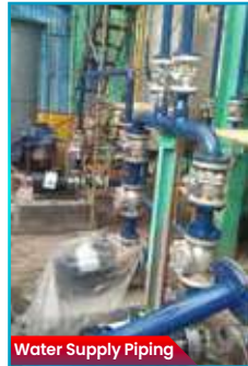
Water Supply Piping
