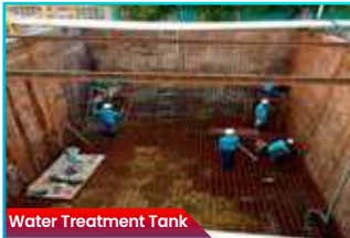
Water Treatment Tank
